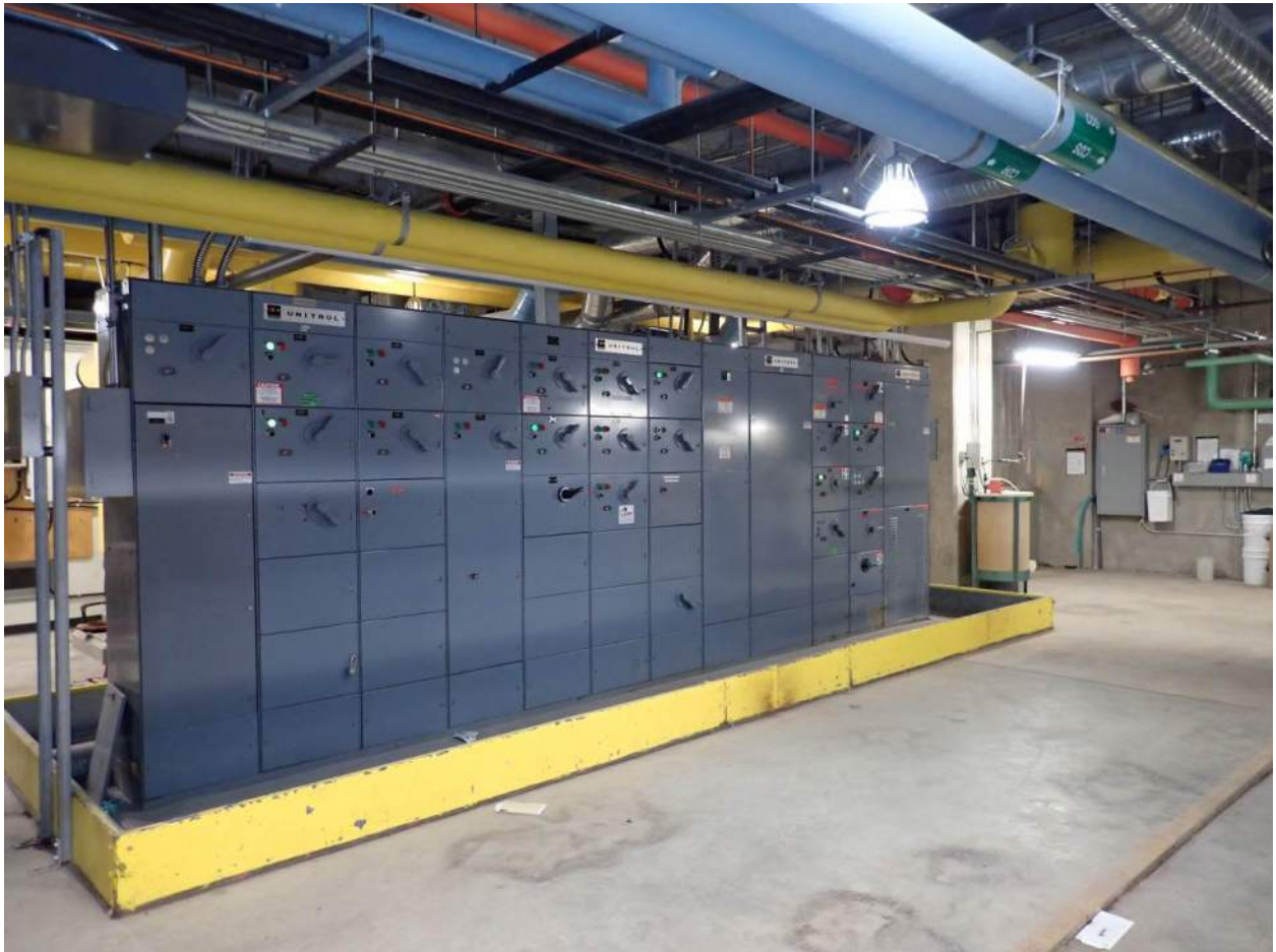
Photo 11 – City Hall MCC
