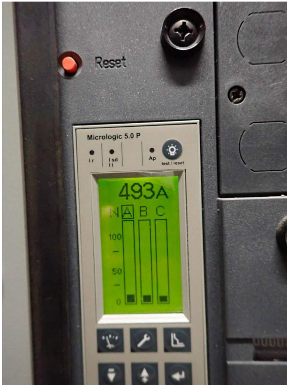
Photo 8 – City Hall Distribution A – Electrical Load on Feb 12, 2021
