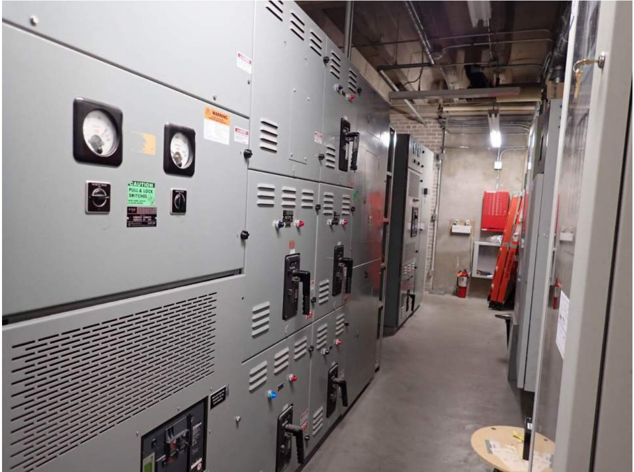
Photo 5 – City Hall Distribution A
