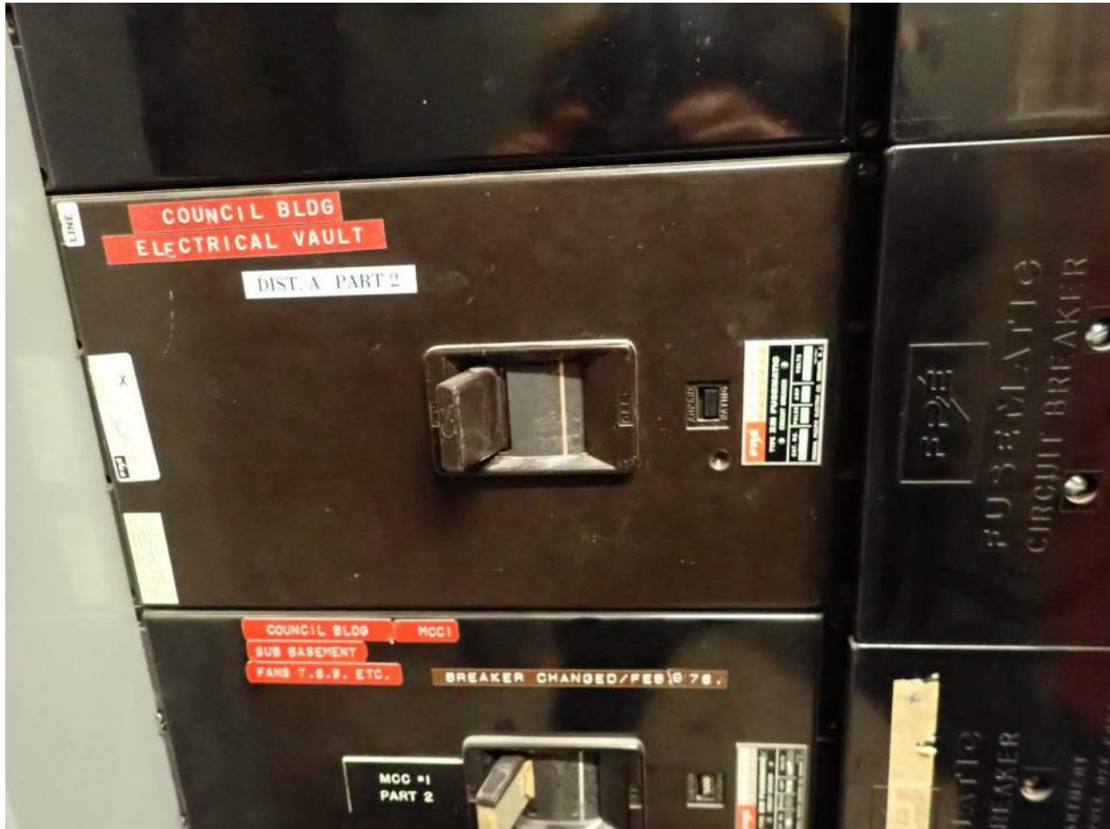
Photo 4 – City Hall Distribution B Breaker Supplying Council Building
