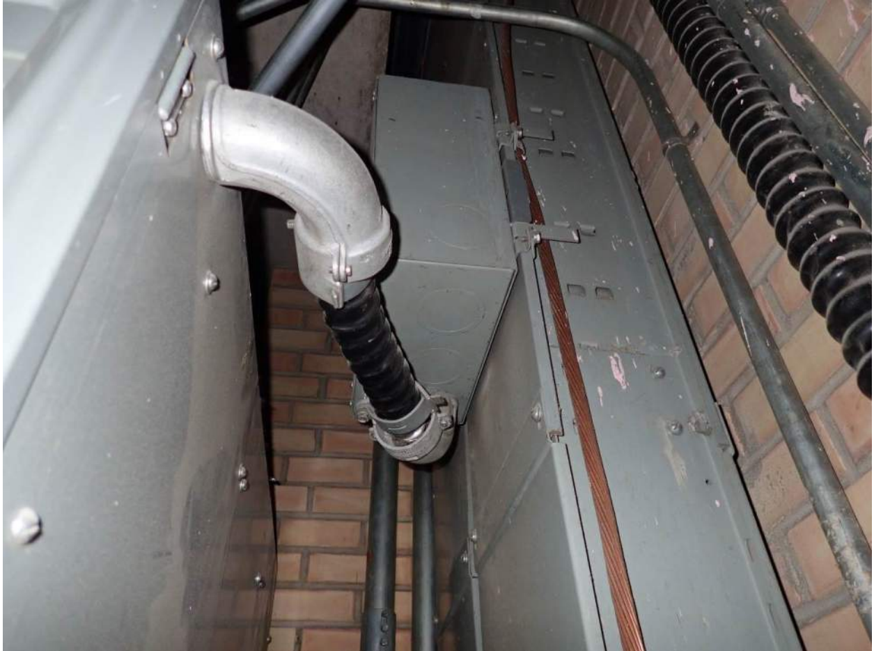
Photo 10 – City Hall Busduct Riser (Typical)
