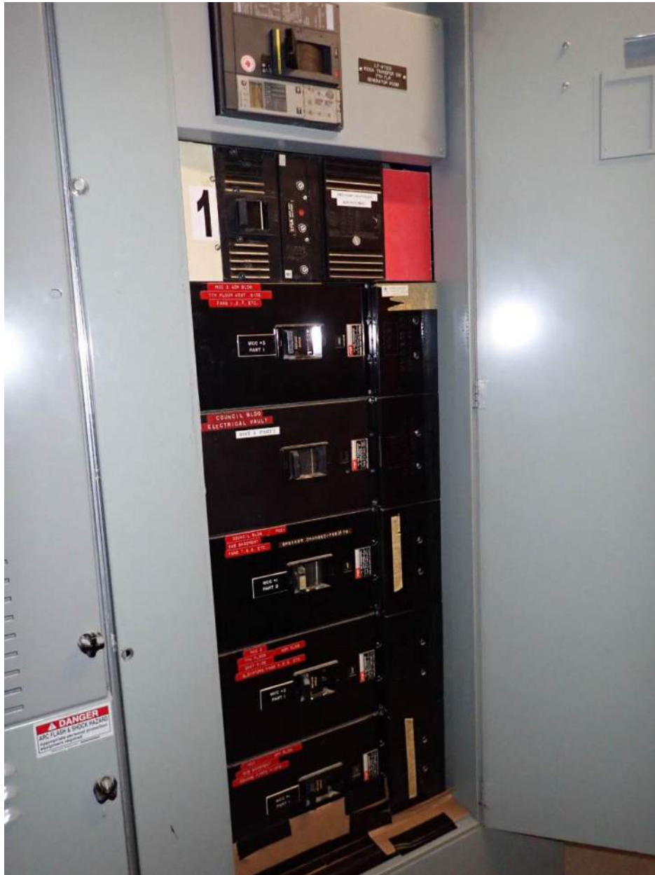
Photo 3 –1200A CDP Section of City Hall Distribution B
