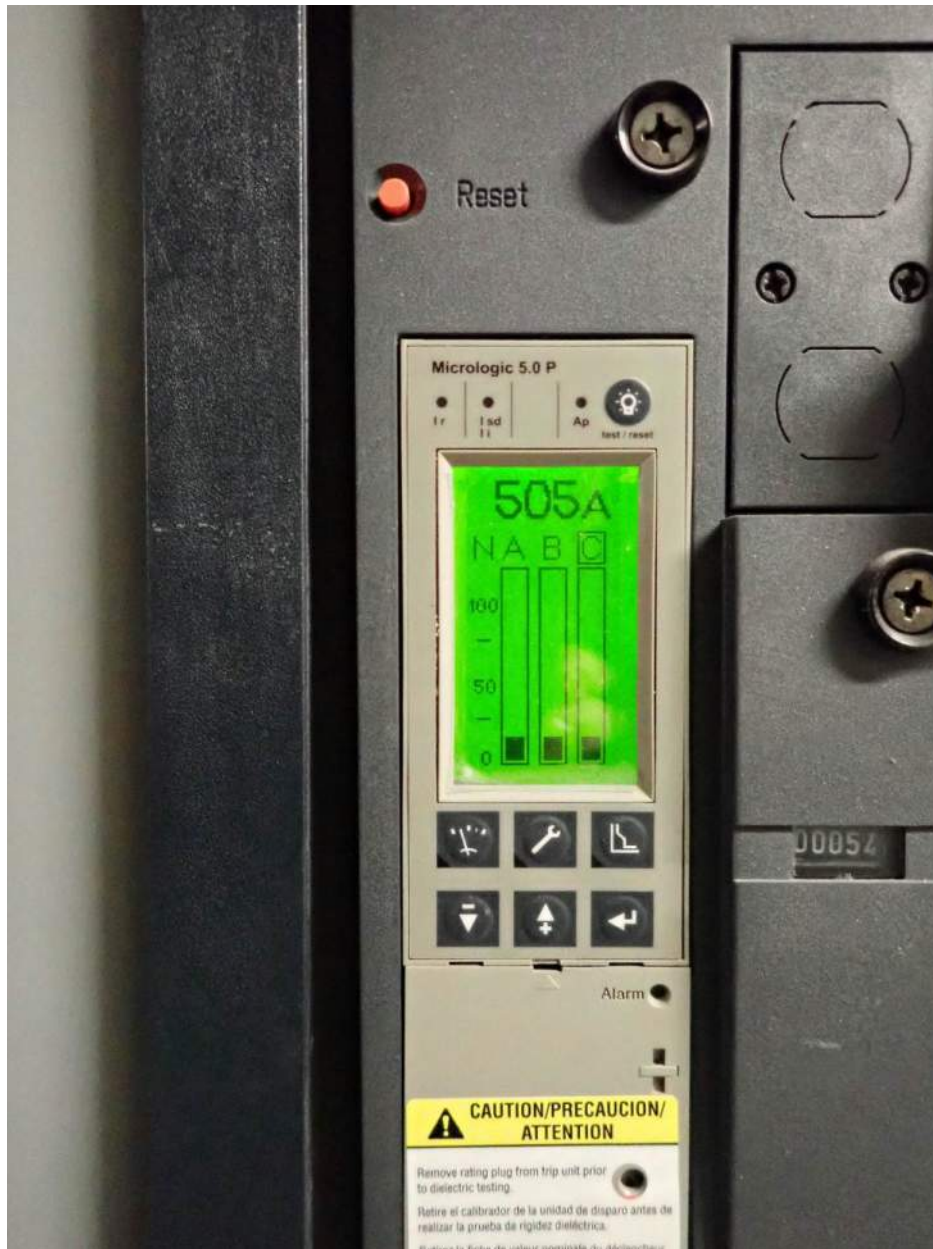
Photo 7 – City Hall Distribution B – Electrical Load on Feb 12, 2021
