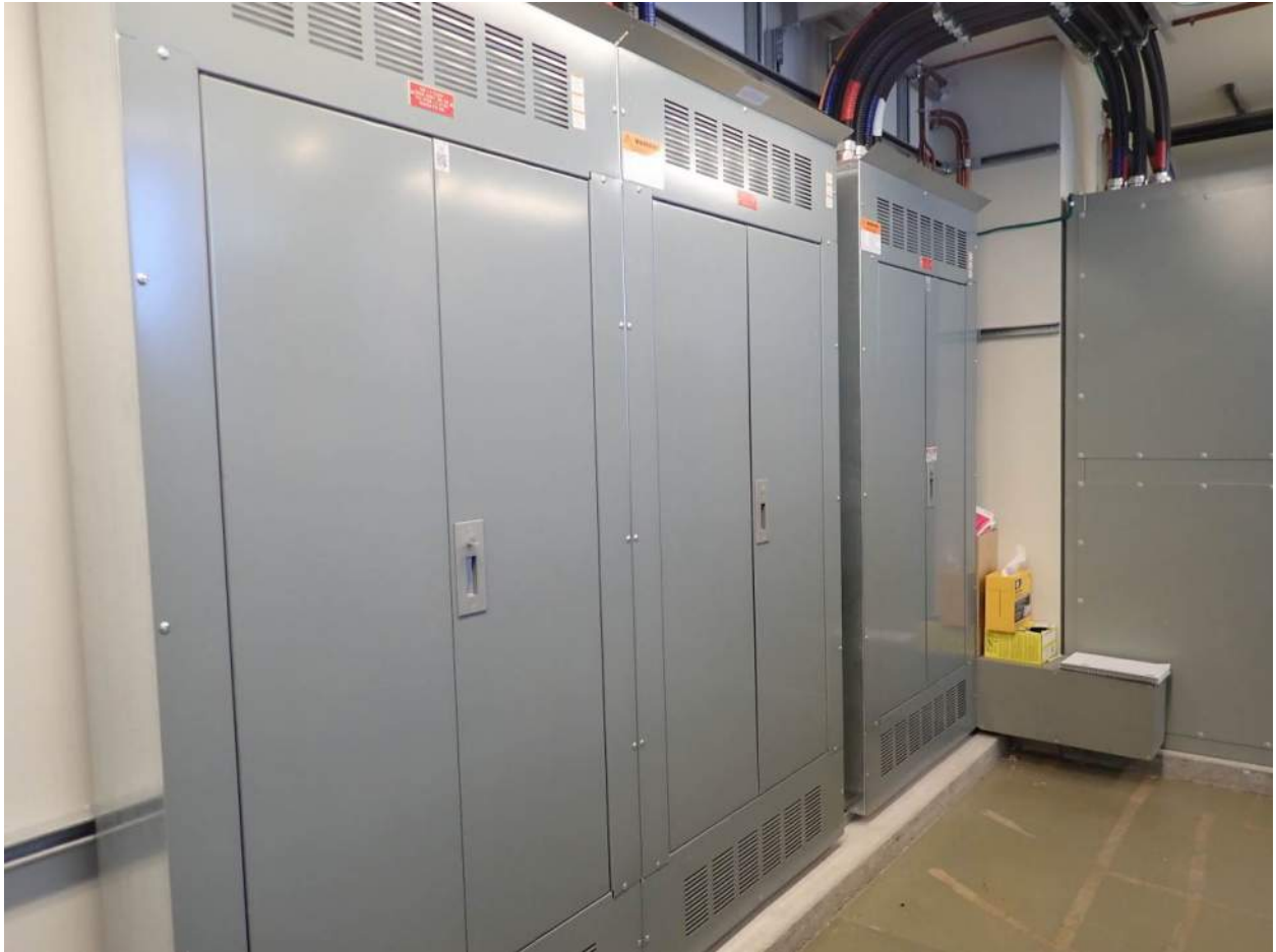
Photo 13 – City Hall Level 7 Emergency Power Distribution
