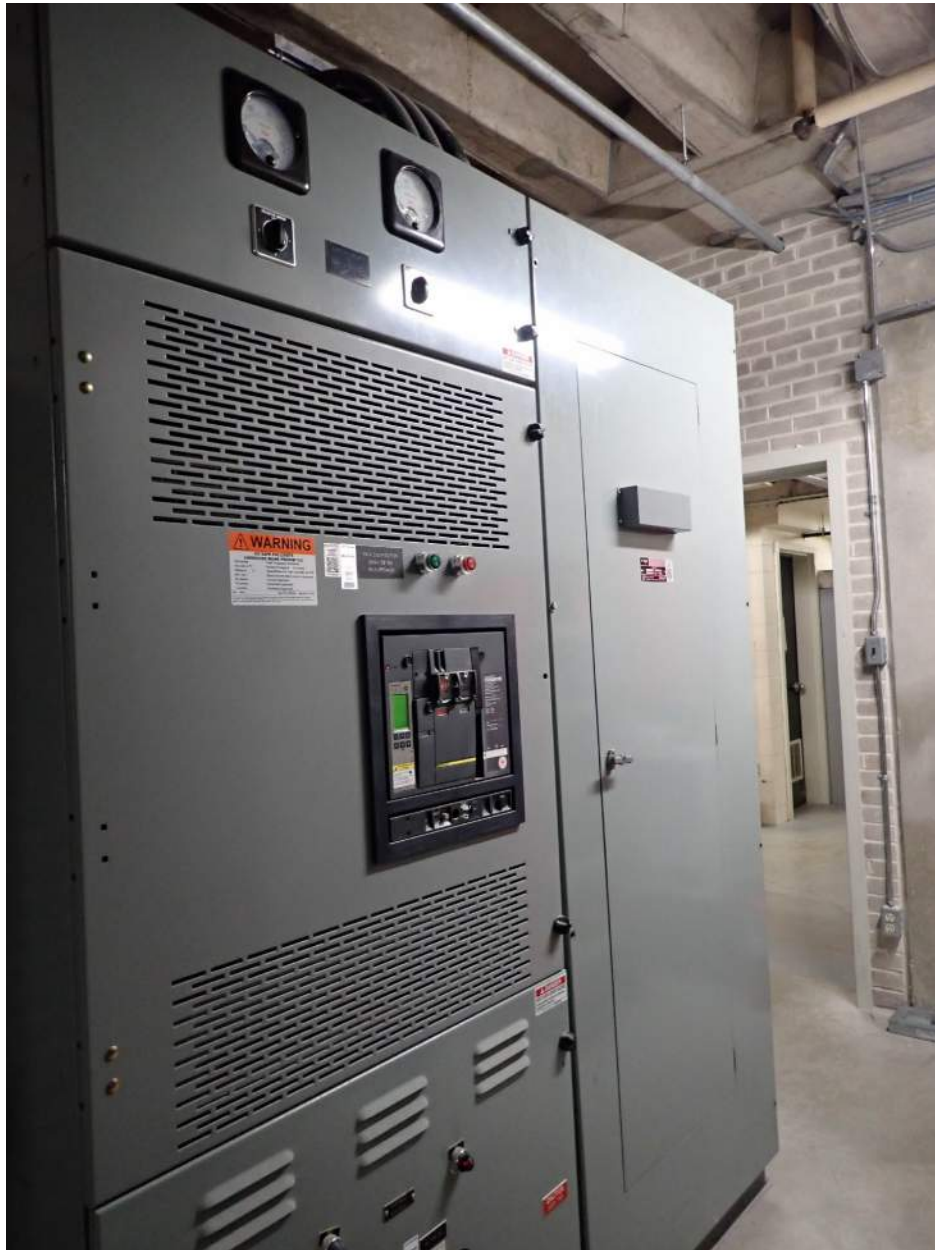
Photo 1 – City Hall Distribution B (600V)
