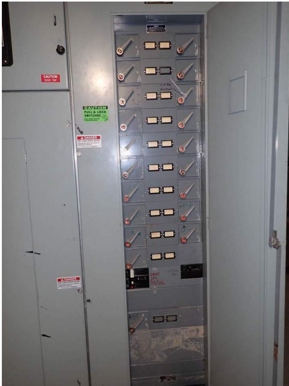
Photo 16 – Council Building Distribution A
