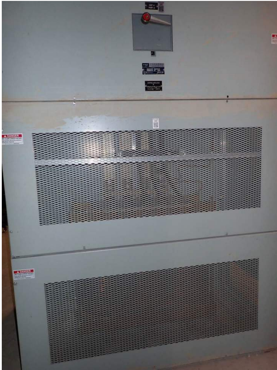
Photo 15 – Council Building Distribution A - Transformer Section
