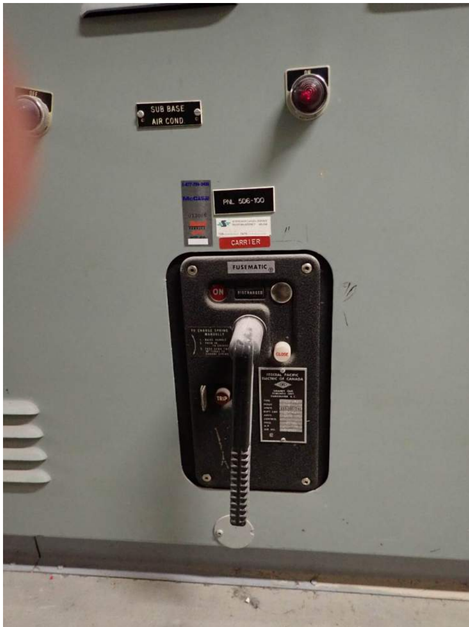
Photo 2 – City Hall Distribution B - Sub-Basement Air Conditioning Breaker
