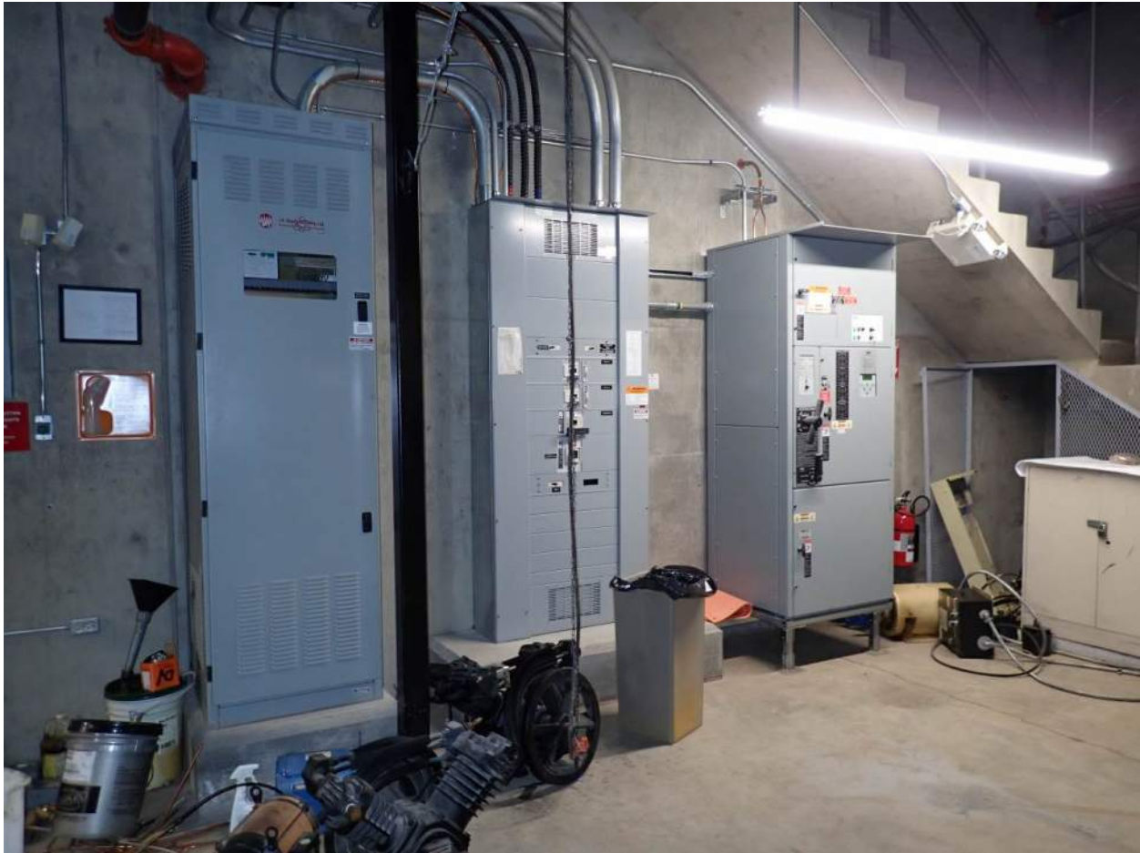
Photo 12 – City Hall Sub-Basement Emergency Power Distribution
