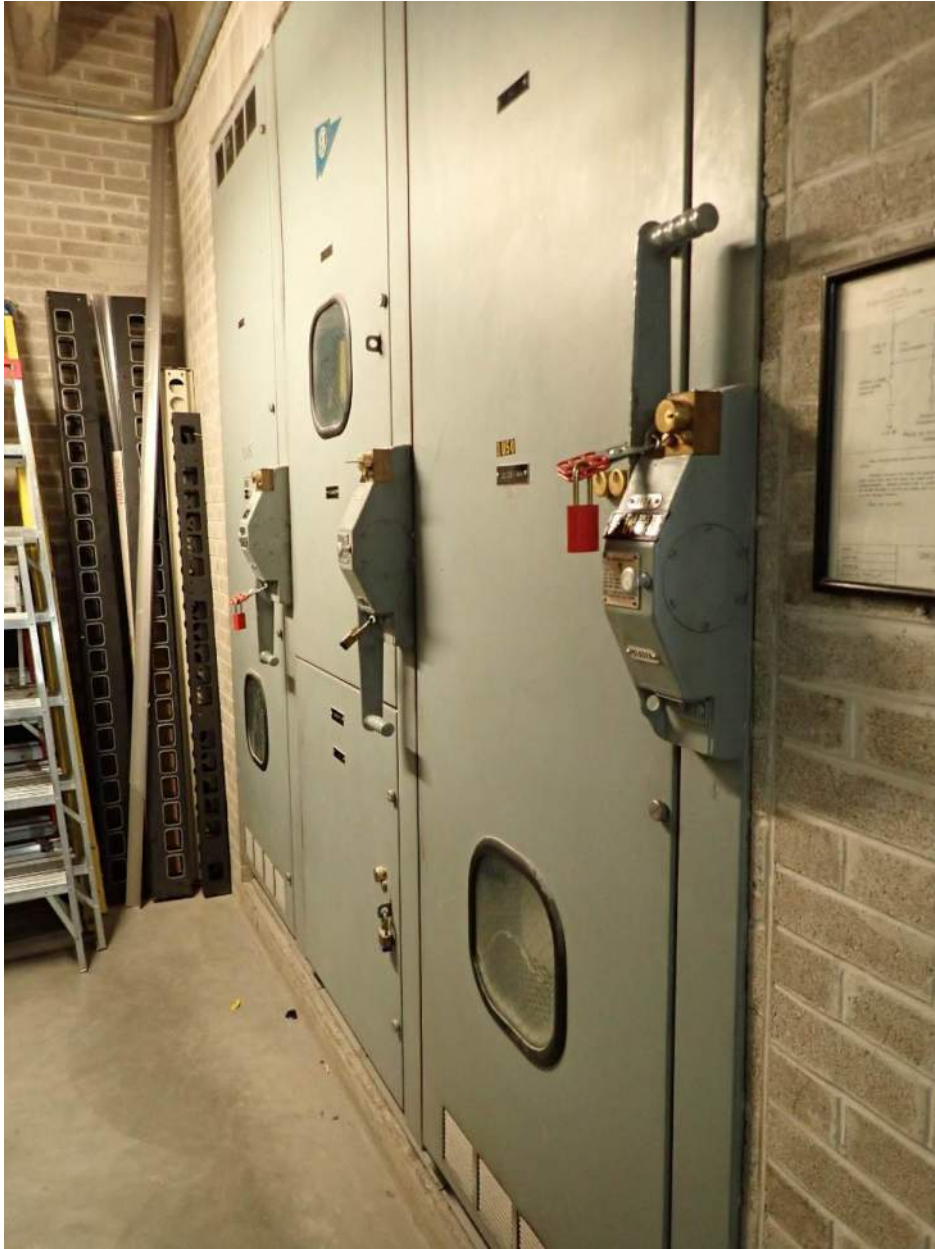
Photo 6 – Electrical Vault in City Hall
